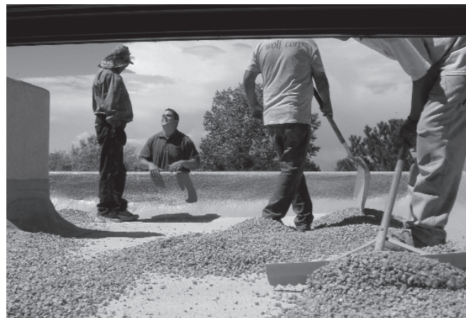
Figure 3. Some roofers protect SPF roofing from ultraviolet light with crushed stone ballast. Stone ballast only works on relatively flat roofs. [Photo credit: Thermal Coatings and Insulation]
