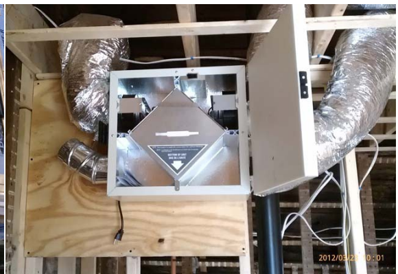
Heat Recovery Ventilation for all units
