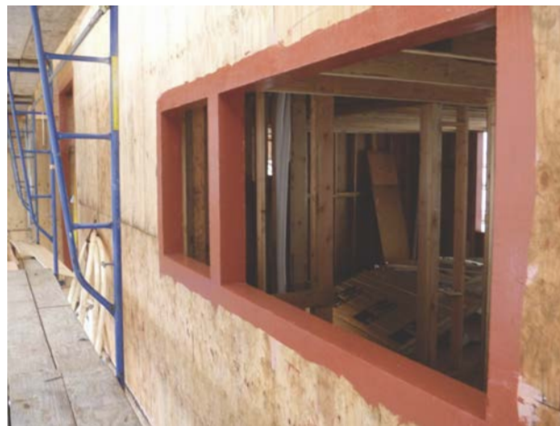
A flashed rough opening awaits weather-resistive barrier and window installation. Photo courtesy of Skylar Swinford, Hammer & Hand.
