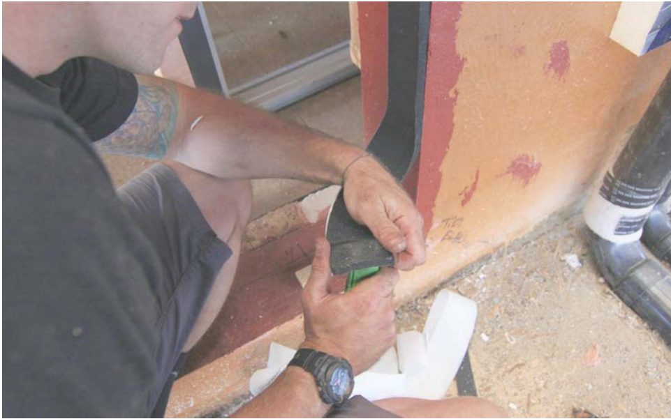
Aaron Quint, Hammer & Hand, installs an expanding foam tape into a flashed doorway rough opening. Under compression, the tape expands to create an airtight, insulated seal that sheds water. Photo courtesy of Skylar Swinford, Hammer & Hand.
