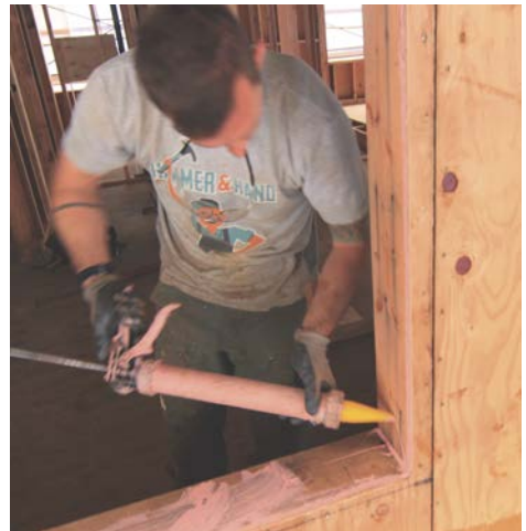
After sanding the rough edges, Aaron Quint, Hammer & Hand, applies a joint-filling compound to seams and penetrations to reinforce against potential movement at joints.
