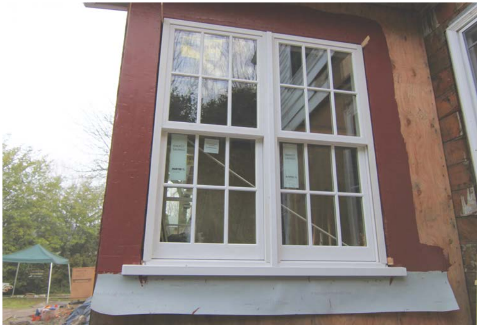
A transition sheet embedded in the flashing helps direct wind-driven water away from the rough opening. Note the liquid flashing extending 9 inches (23 cm) around the window to gasket fastener penetrations and protect against wind-driven rain that can migrate horizontally past the WRB. Photo courtesy of Skylar Swinford, Hammer & Hand.
