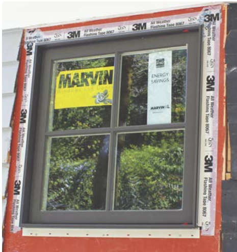
Flexible nailing flanges, or fins, on some windows can be hard to embed in a liquid flashing system. Here, a weather-resistive tape provides an additional layer of protection over the nail heads. Photo courtesy of Skylar Swinford, Hammer & Hand.
