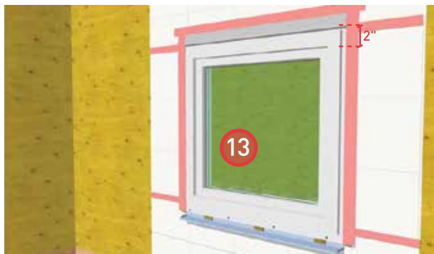
13. Install metal flashing at the head of the window. Seal the leading edge of the flashing with sheathing tape.
