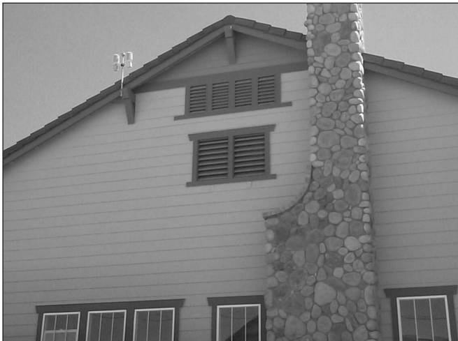
Figure 3. In this photo, the NightBreeze air intake grille is behind the lower set of louvers.
