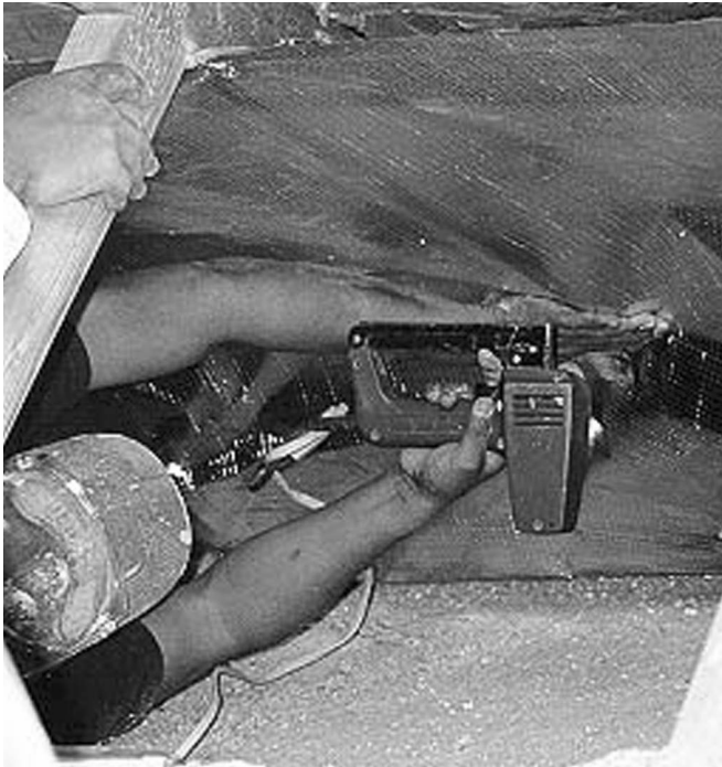
Figure 6 — Installation of the attic radiant barrier was particularly awkward near the eaves.
