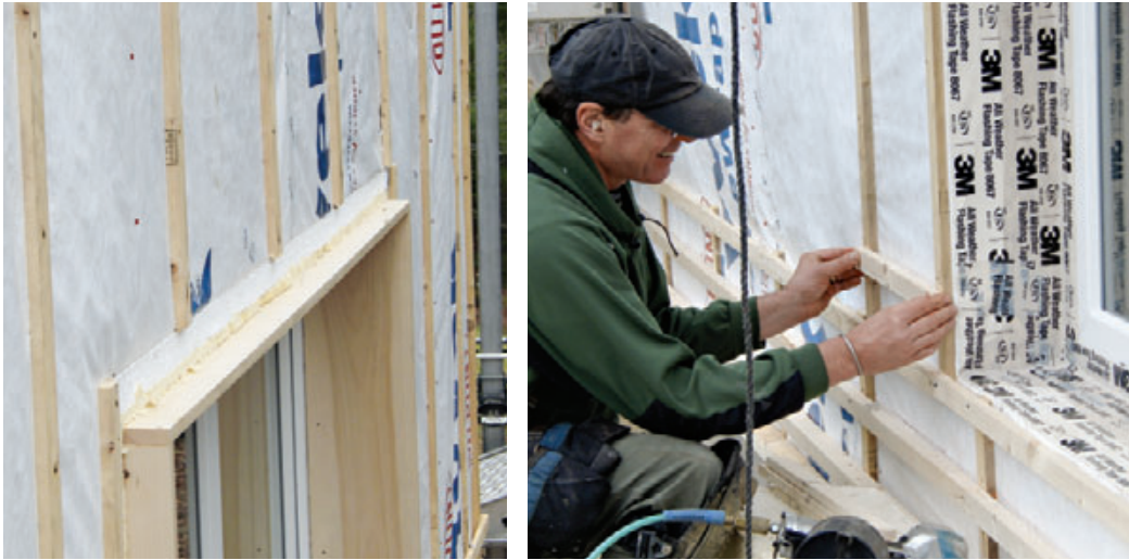
Figure 7. Vertical furring strips cut on site from framing lumber (far left) promote drying behind the pine clapboards. Additional horizontal furring provides backing for cedar shakes at the base of the wall (left).
