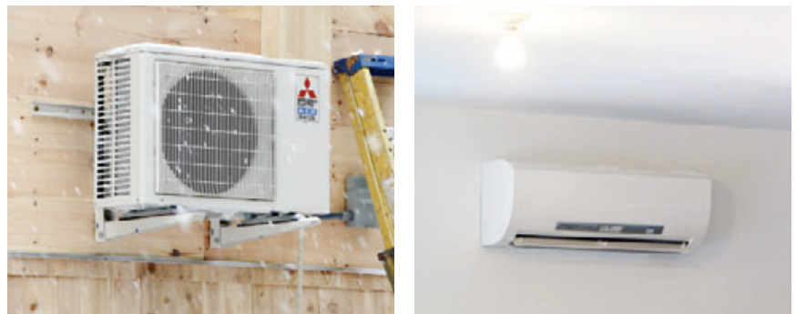
Figure 10. A 12,000-Btu Mitsubishi mini-split heat pump provides heating and cooling (left). A single indoor unit (right) delivers the warm air, which will be further circulated by the ERV ductwork.
