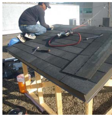
Figure 7: Three-tab asphalt shingles being installed by roofing contractor over #15 felt or SAM at the control roof.
