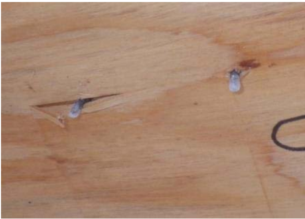
Figure 17: Frost on nail heads of south-facing roof slope on morning of January 2, 2013
