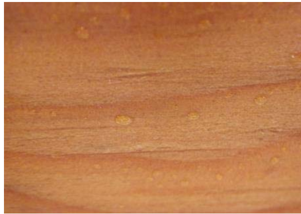
Figure 18: Condensation on underside of plywood sheathing on morning of January 2, 2013. Note that surface condensation at this time only occurred on certain areas of the plywood and was affected by wood grain.
