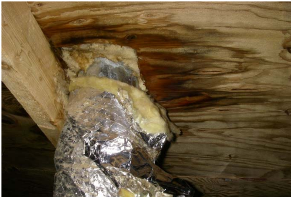
Figure 3: Locally stained, wet, and deteriorated sheathing from water ingress around a plugged dryer exhaust duct boot
