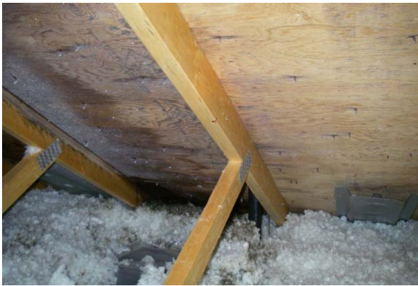
Figure 1: Locally stained and wet sheathing and frost due to condensation of humid air leaking from a poorly sealed bathroom exhaust fan and duct.
