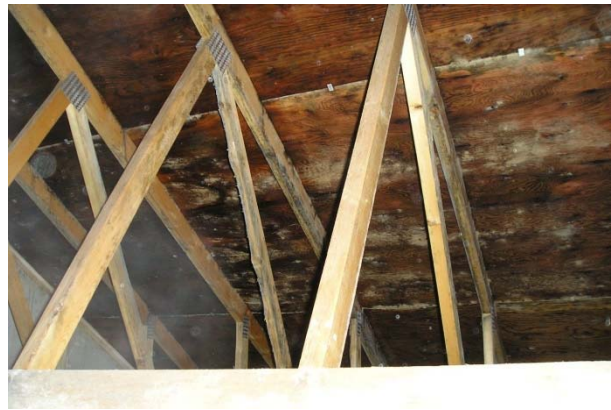
Figure 2: A wood frame attic with widespread stained, wet, and deteriorated sheathing from persistent indoor and exhaust duct air leakage and poor attic ventilation
