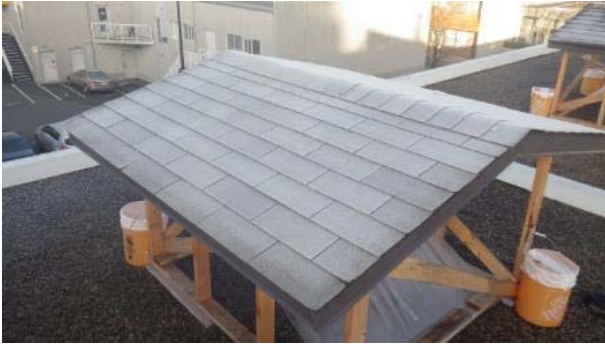
Figure 15: Frost on exterior of shingles during morning of January 2, 2013
