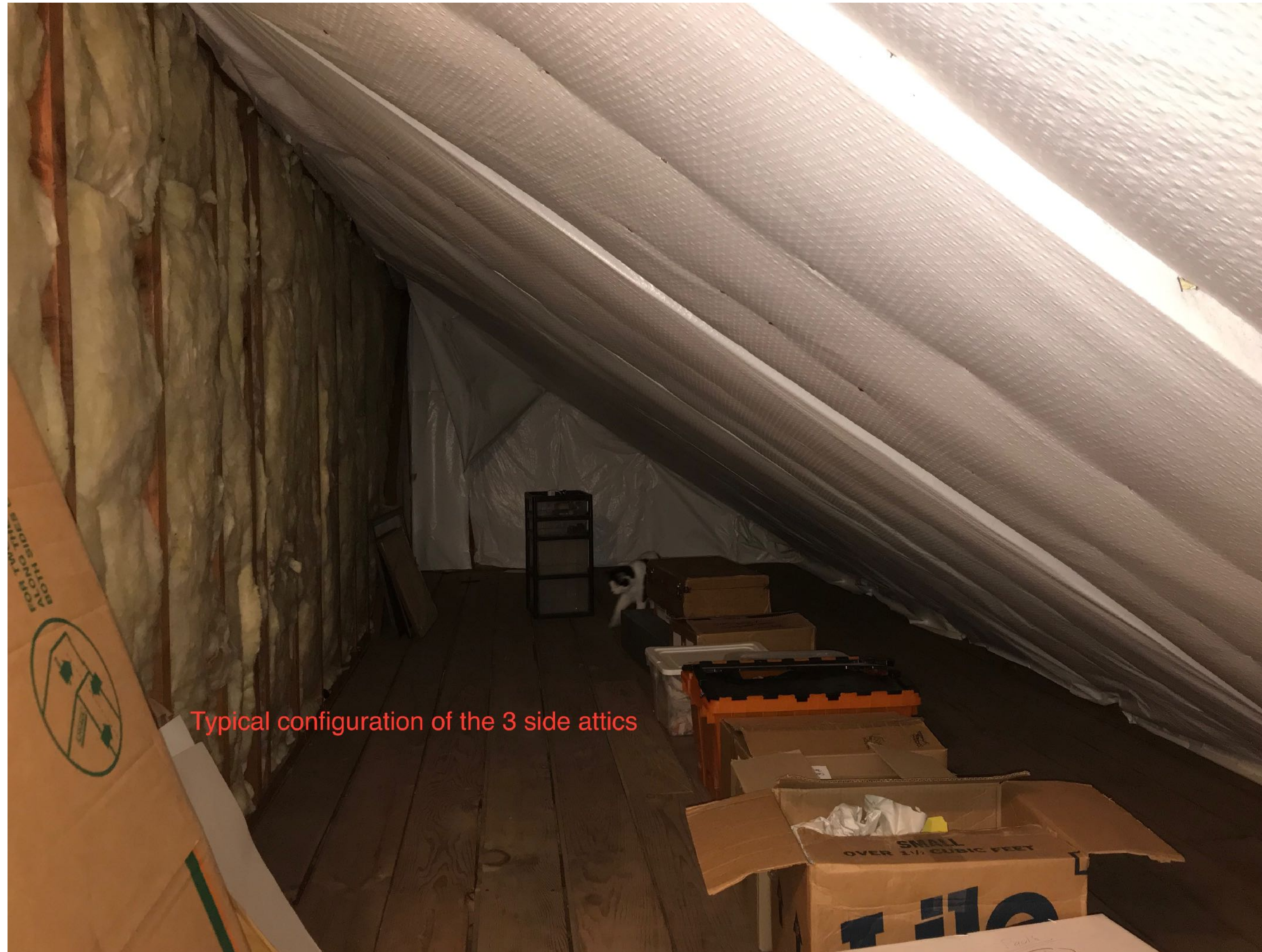
Initial configuration showing vinyl on the rafters and the knee wall insulation
