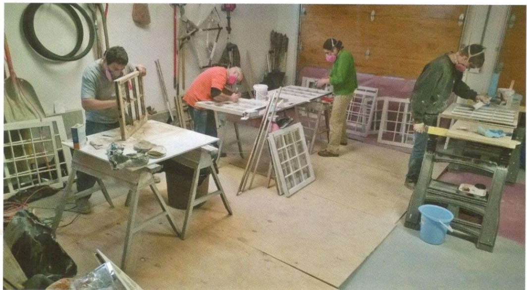
FIGURE 1: THE AUTHOR'S CREW RESTORING WOOD WINDOWS, A LABOR INTENSIVE TASK. CREDIT: ALL PHOTOS BY AUTHOR
