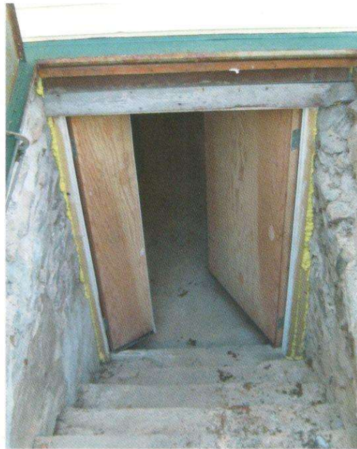
FIGURE 2: SITE BUILT INSULATED DOOR AT THE BOTTOM OF THE BASEMENT BULKHEAD.
