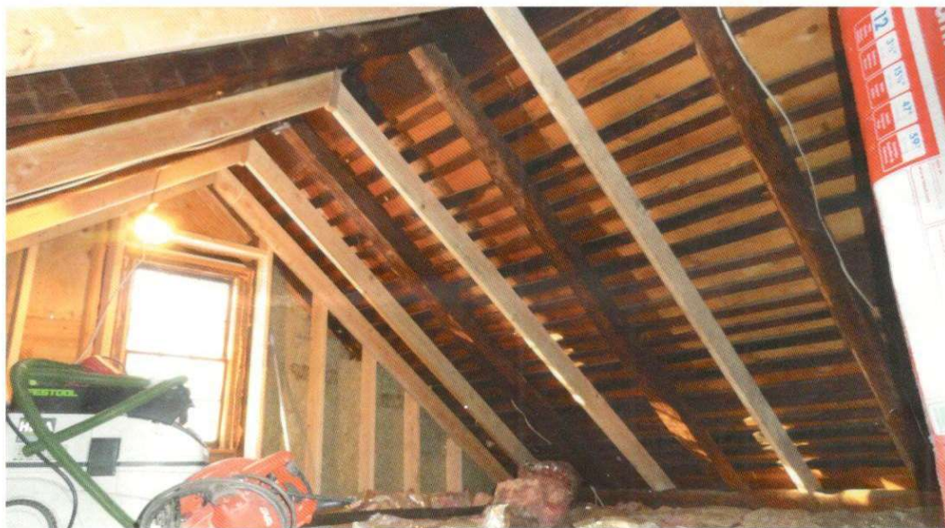
FIGURE 3: NEW RAFTERS ADDED BETWEEN ORIGINAL TIMBER RAFTERS MAKE IT SIMPLE TO INSTALL ROCKWOOL BATTS.
