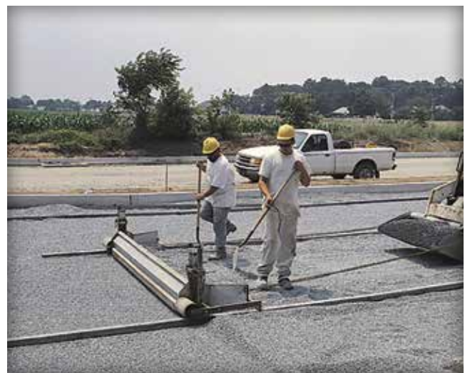
Figure 25. A screed beam pulled by equipment can be more efficient and productive.
