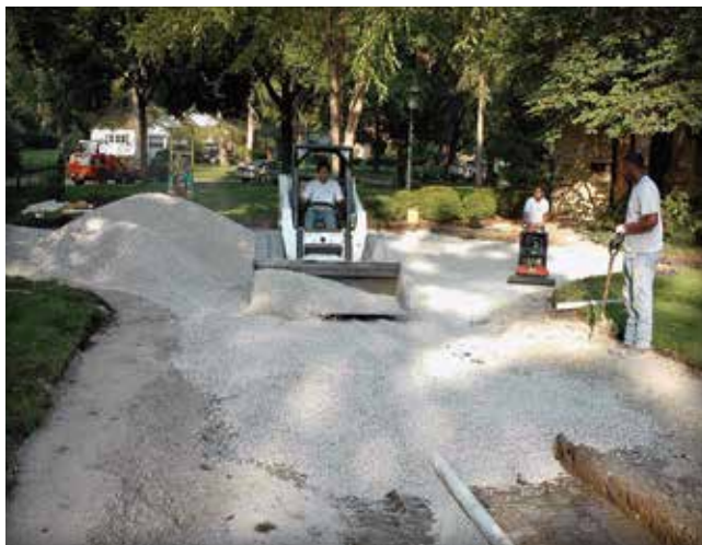
Figure 17. Perimeter berms made with dense-graded base are in place prior to placing open-graded aggregate in the driveway.
