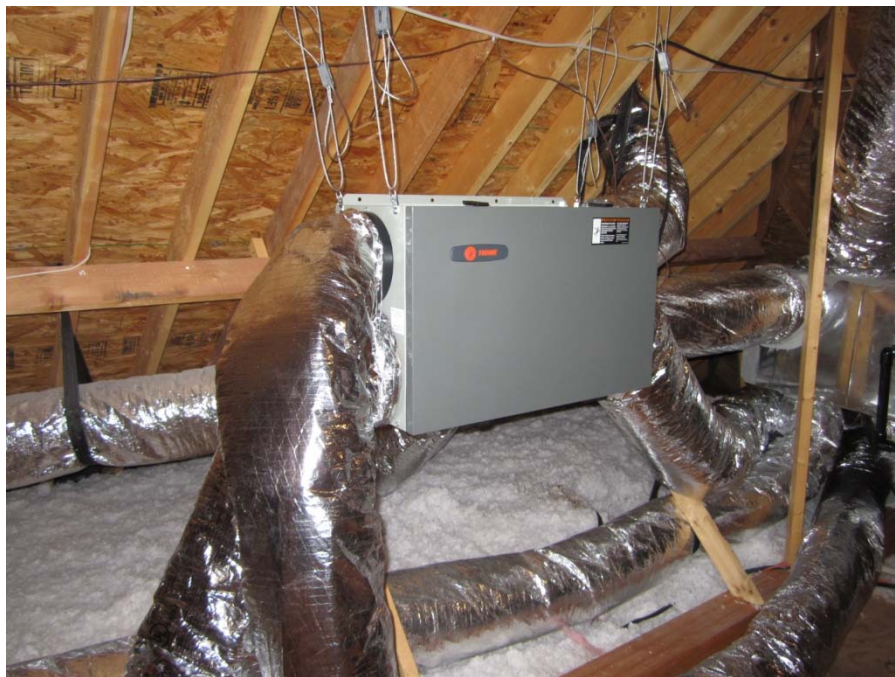
Figure 8. Energy Recovery Ventilator installed in House 1 to match that of House 2
