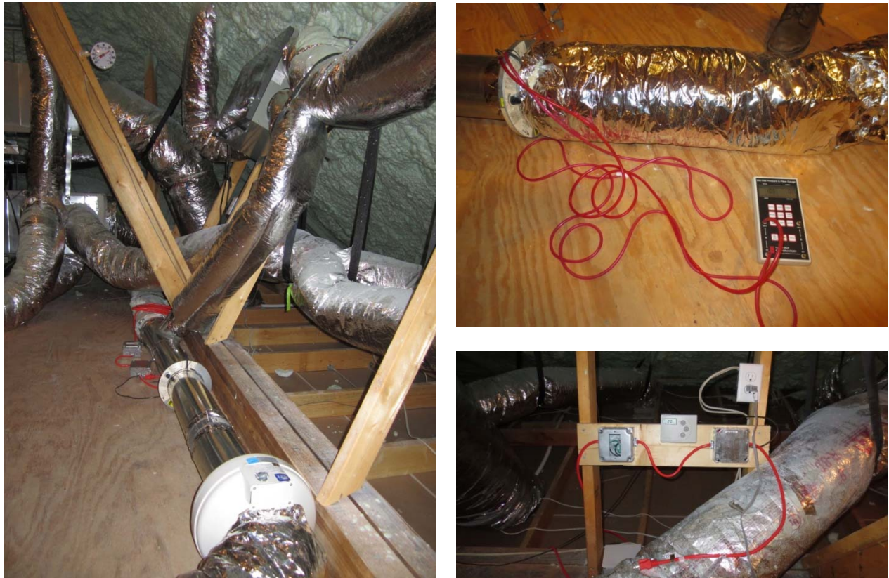
Figure 9. Wye'd outside air duct, airflow stations, and inline fan for retrofitting a CFIS ventilation system in each attic (left); setting the CFIS airflow rate with Iris damper airflow station (top); fan timer and relay arrangement (bottom)
