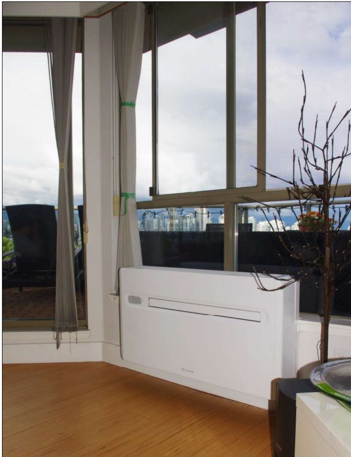
Innova 2.0 unit installed in a condo unit at the Meridian Cove.
