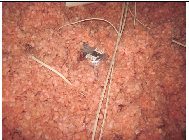
Figure 28-Insulation covering IC light?
