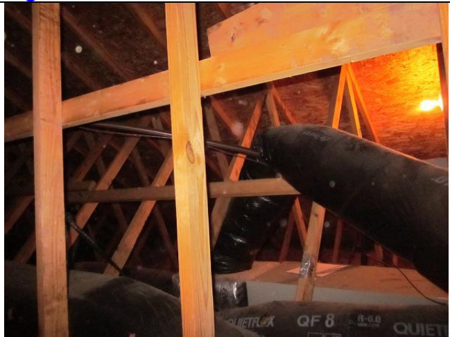
Figure 5-Trunk line bent at 90 degrees.
