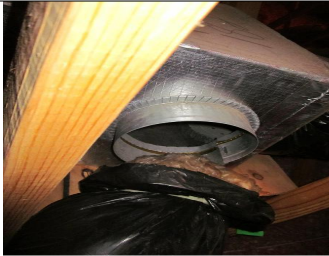
Figure 3-Trunk lines disconnected in attic.
