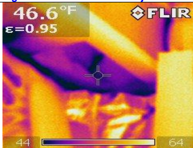
Figure 15-IR image of rim band joist.
