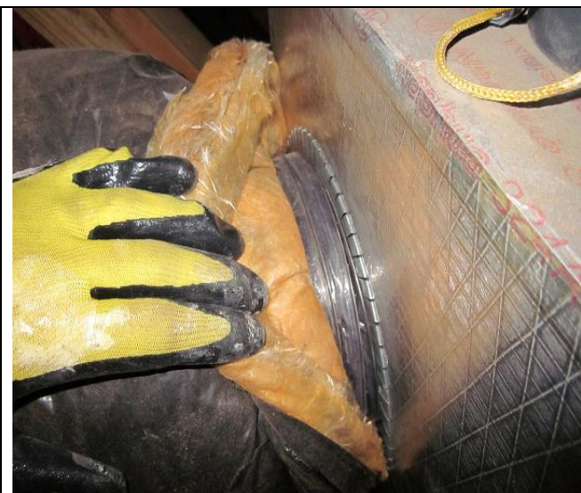
Figure 1-Air leaking out around collars.
