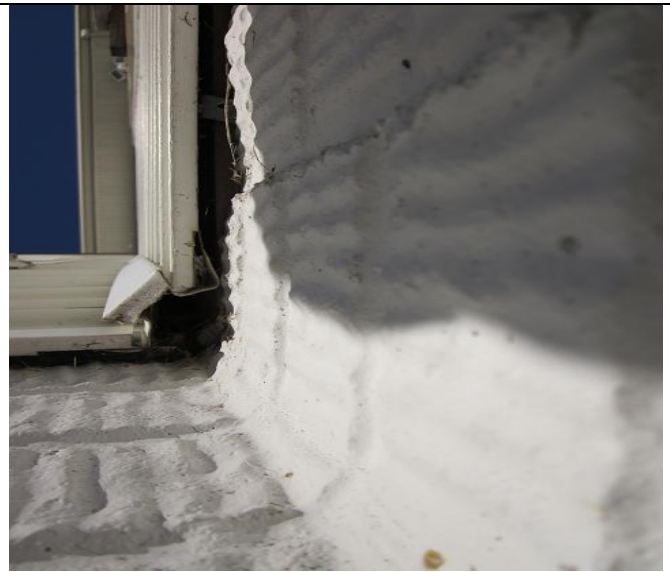
Figure 10-Air moving under siding.
