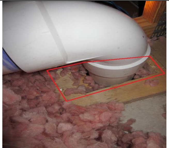
Figure 22-Fresh air exhaust vent hole.
