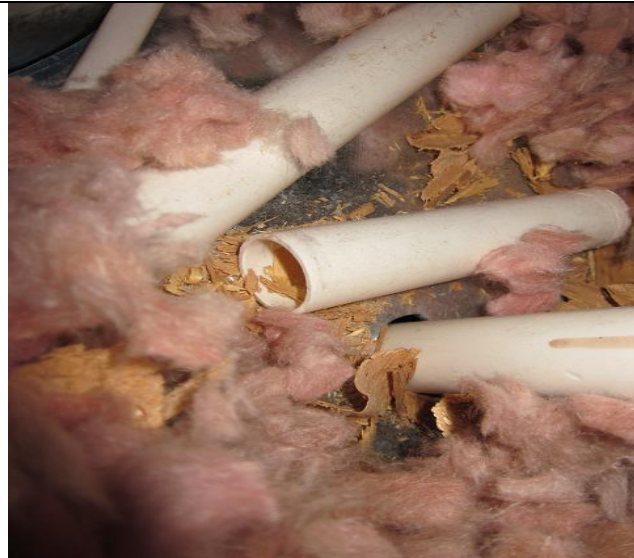
Figure 29-Holes with no wires.
