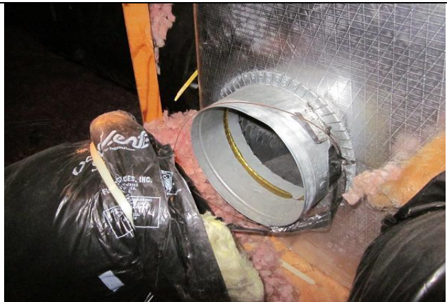
Figure 7-Open flexible supply duct line.
