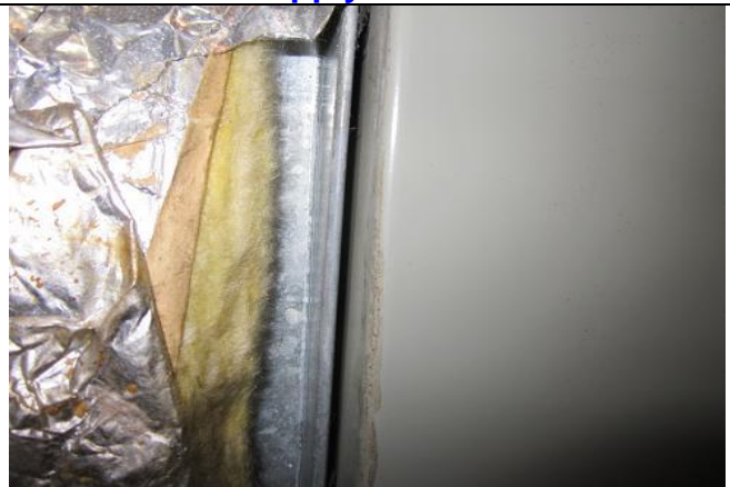
Figure 8- Plenum not taped to air handler.
