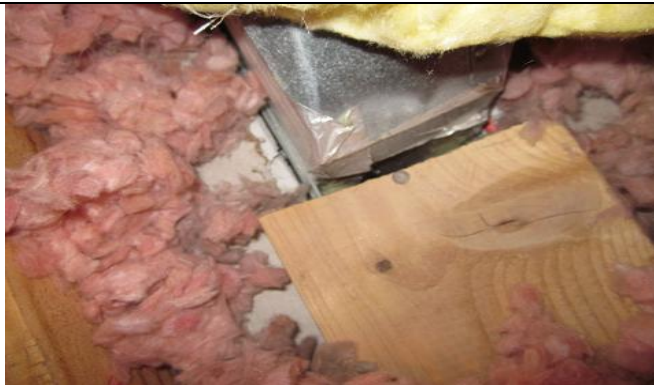
Figure 7-Duct vent not sealed to ceiling
