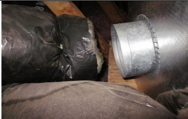
Figure 5-Collar and duct connections with no mastic or tape.
