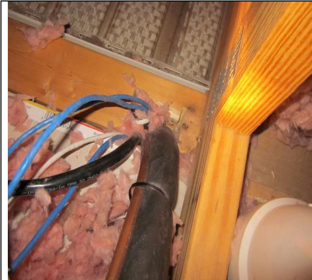
Figure 21-Hole in top plate in attic.
