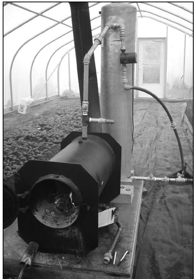
Figure 7. Lehman's Hardware sells a wood-fired water heater made of ¾-inch-thick welded steel. Although this photo shows a greenhouse installation, the water heater is typically installed in a basement.
