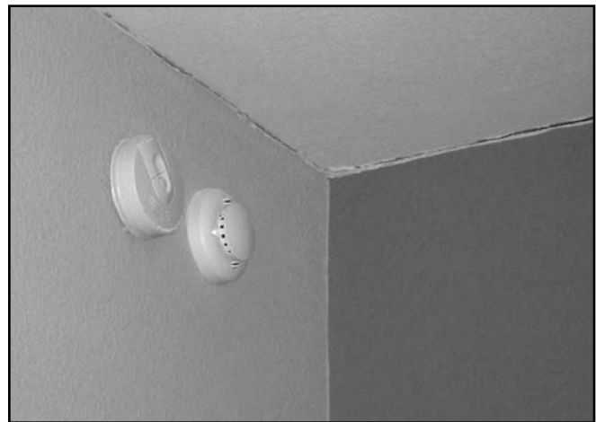
Figure 2. Usually, the first sign of the white-roof problem is cracked drywall caused by truss uplift.
