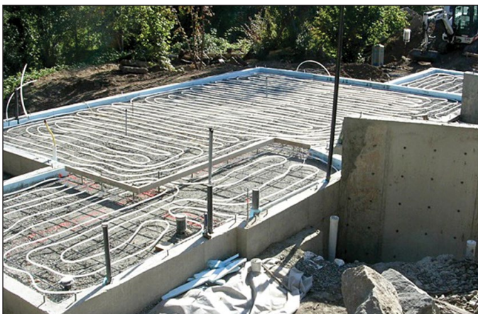
Below: compacted gravel and hydronic heating tubing in place over perlite bag insulation; ready to pour the concrete floor.
